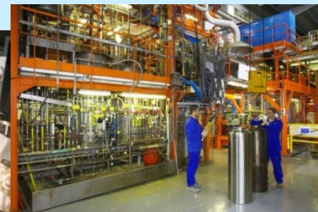
General view of the evolving vitrification prototype equipped with a cold crucible melter adapted for nuclear environments at Marcoule
