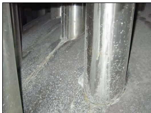
Reactor Vessel Head
