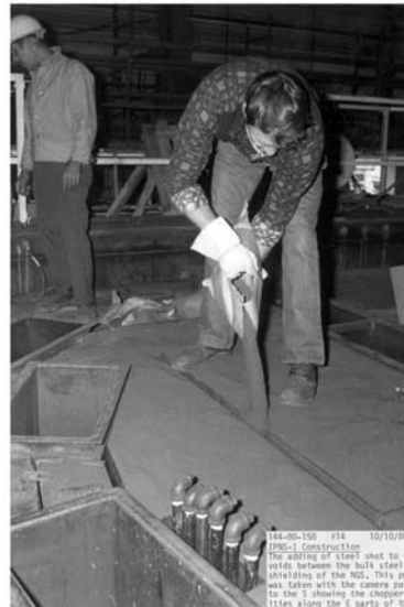
144-00-114 29 8/21/90 IPNS-1 Construction Installation of bulk shielding on the NE corner of the facility near the chopper exit line for beam lines F1 and F2 both of which may be seen in this picture.
