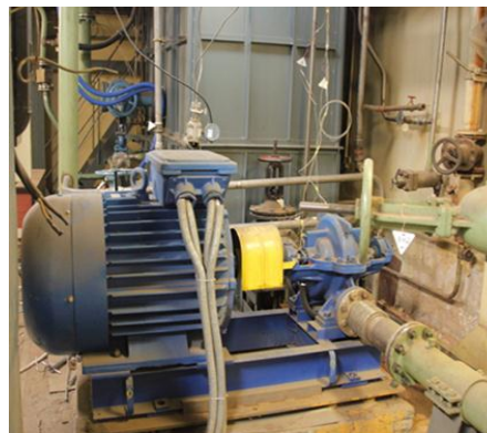
NIKIET: Water High Pressure Stand SVD-2 Large Hydraulic Test Bench (LHTB)
