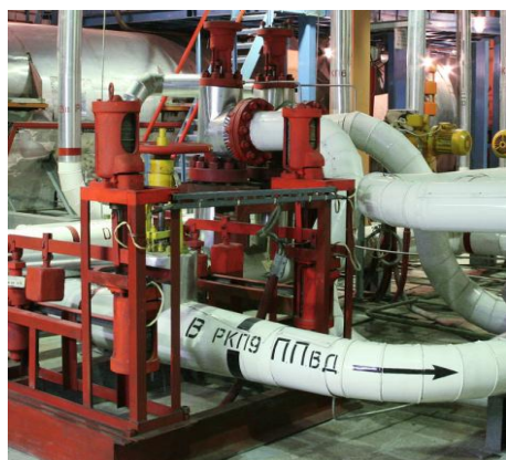
OKBM (He): High-Temperature Gas Facility
