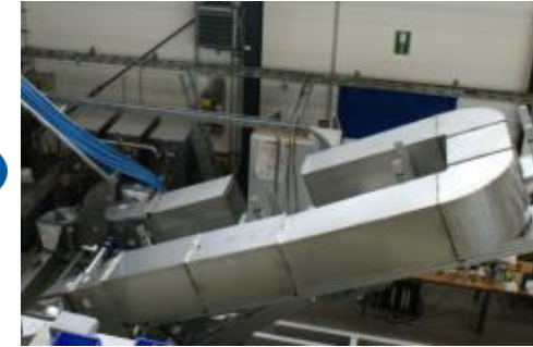
SETCOM : Wall condensation
