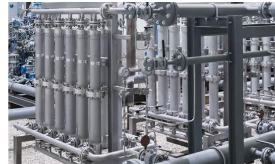
Membrane unit of the laboratory-scale test facility
