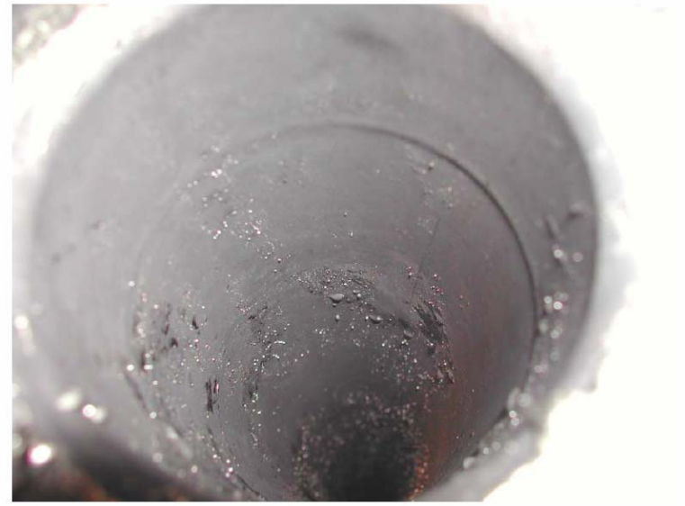
Fig. 4(b). Interior of the pipe after the second run at a higher oxygen concentration.
