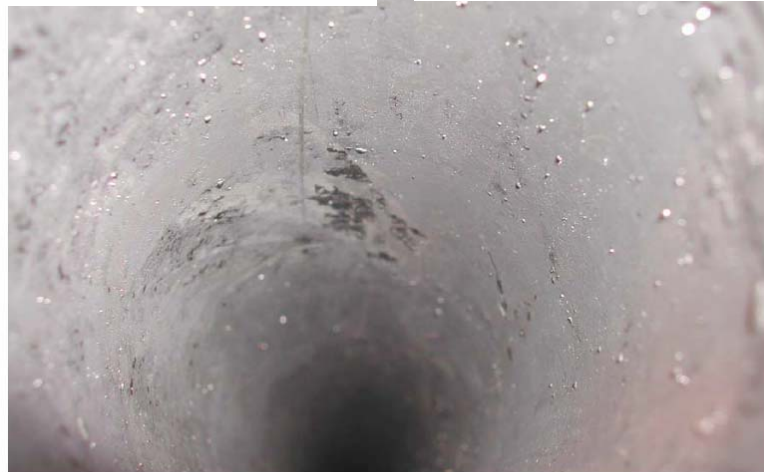
Fig. 4(c). Interior of the pipe after the third run at the highest oxygen concentration, showing significant oxidation and evidence of non-wetting.
