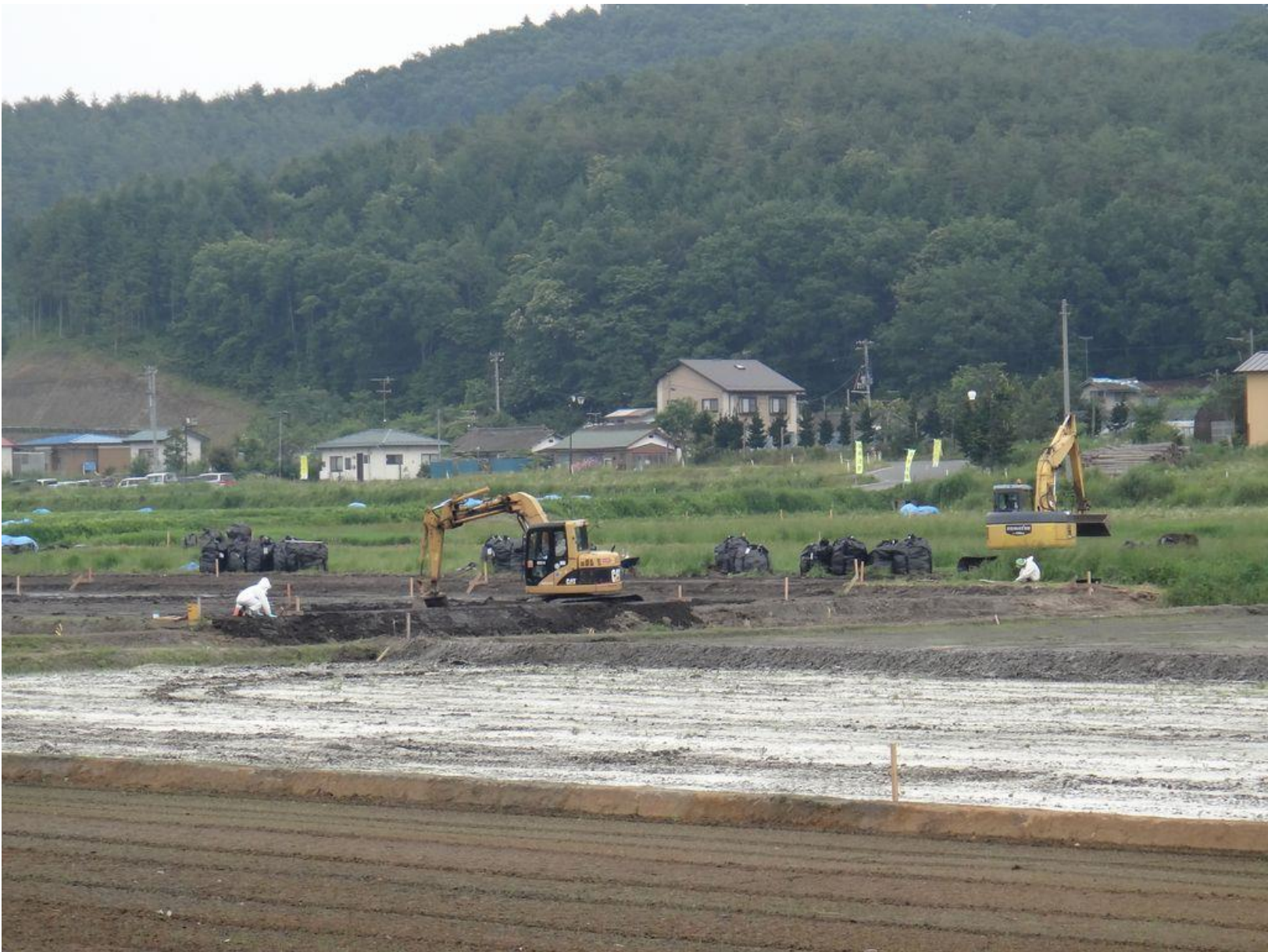
Scraping off decontamination work of surface soil in the “zones preparing for the lifting of the evacuation order” (Iitate village)
