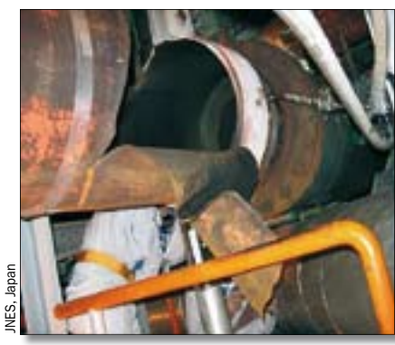
View of a pipe failure.
