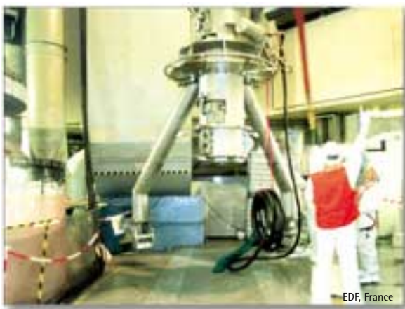
In-service inspection robot at the Bugey nuclear power plant in France.
